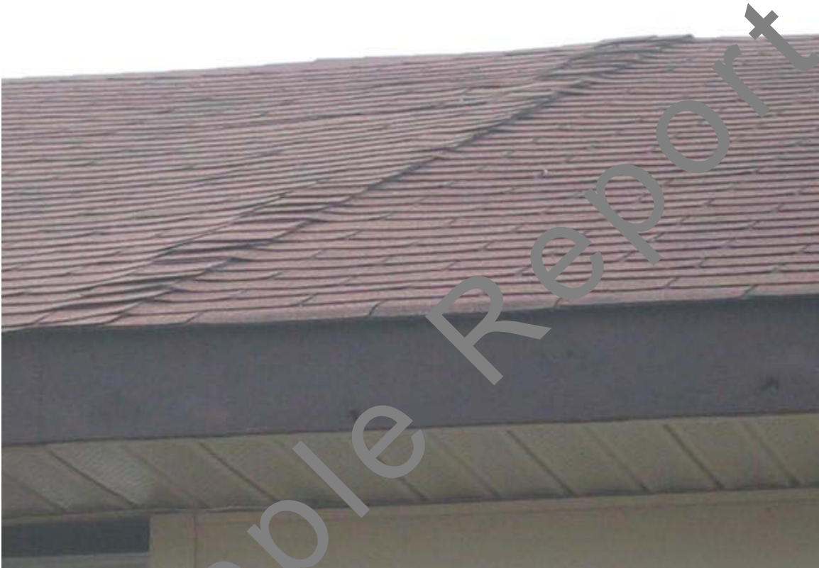
Hump in the roofing shingles over the breezeway.
